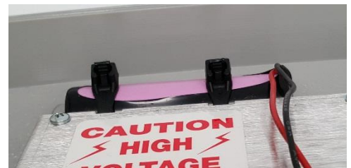
WRONG! Do Not Position Cable Ties Connection on Front of Batteries.
