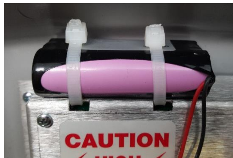
CORRECT! Position Cable Ties Connection on Top of Batteries.
